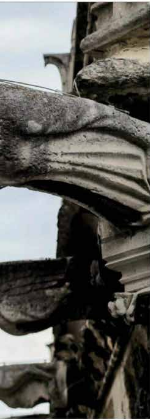
Many of Notre Dame's gargoyles, which act as rain spouts, have corroded and been replaced with PVC tubes
